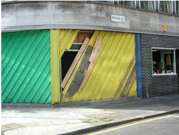
Hoardings ripped apart to gain access to a crack house.
